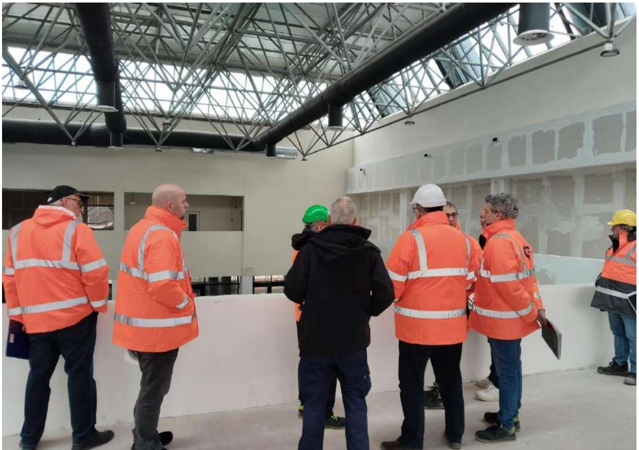
Ongoing finishing and retrofit works of Fushë Kosovë station for both interior arrangements and finishings and external façade and roofing.
