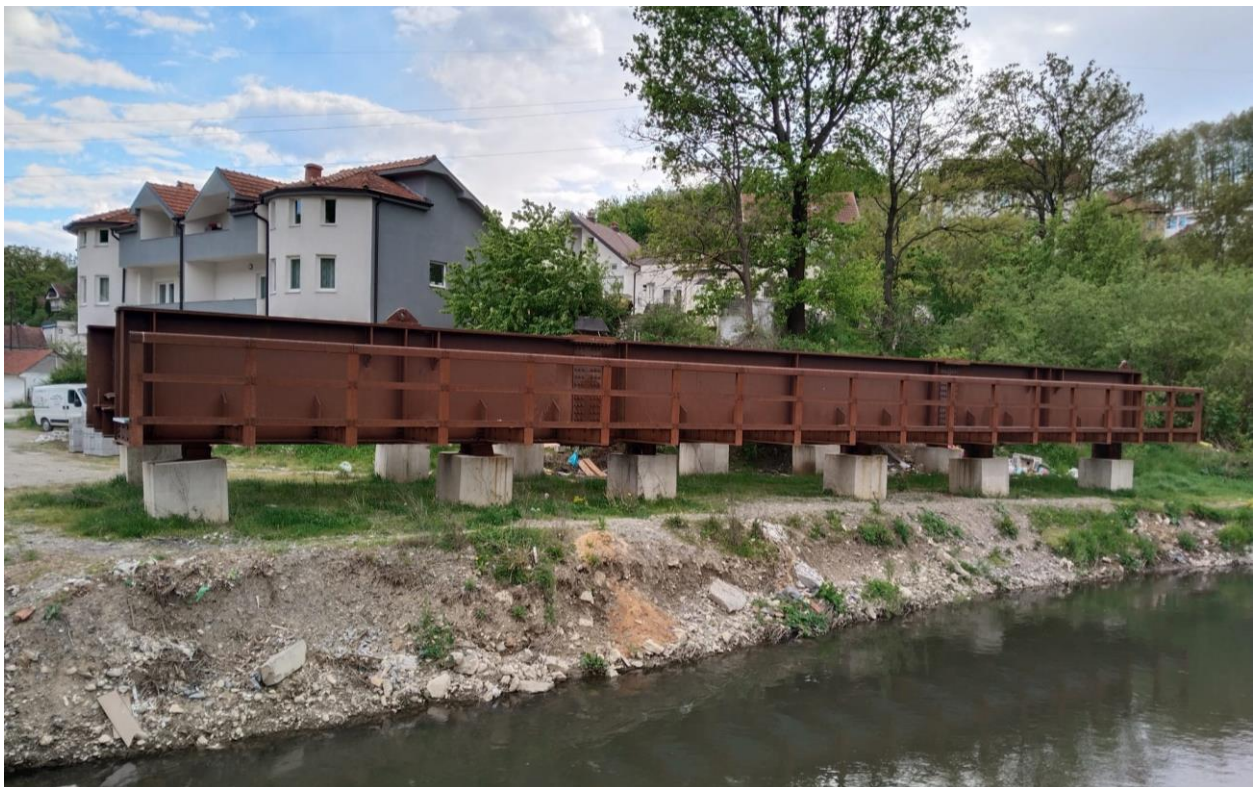
Figure 3 One of the two new Steel Bridges manufactured and delivered by the Contractor
