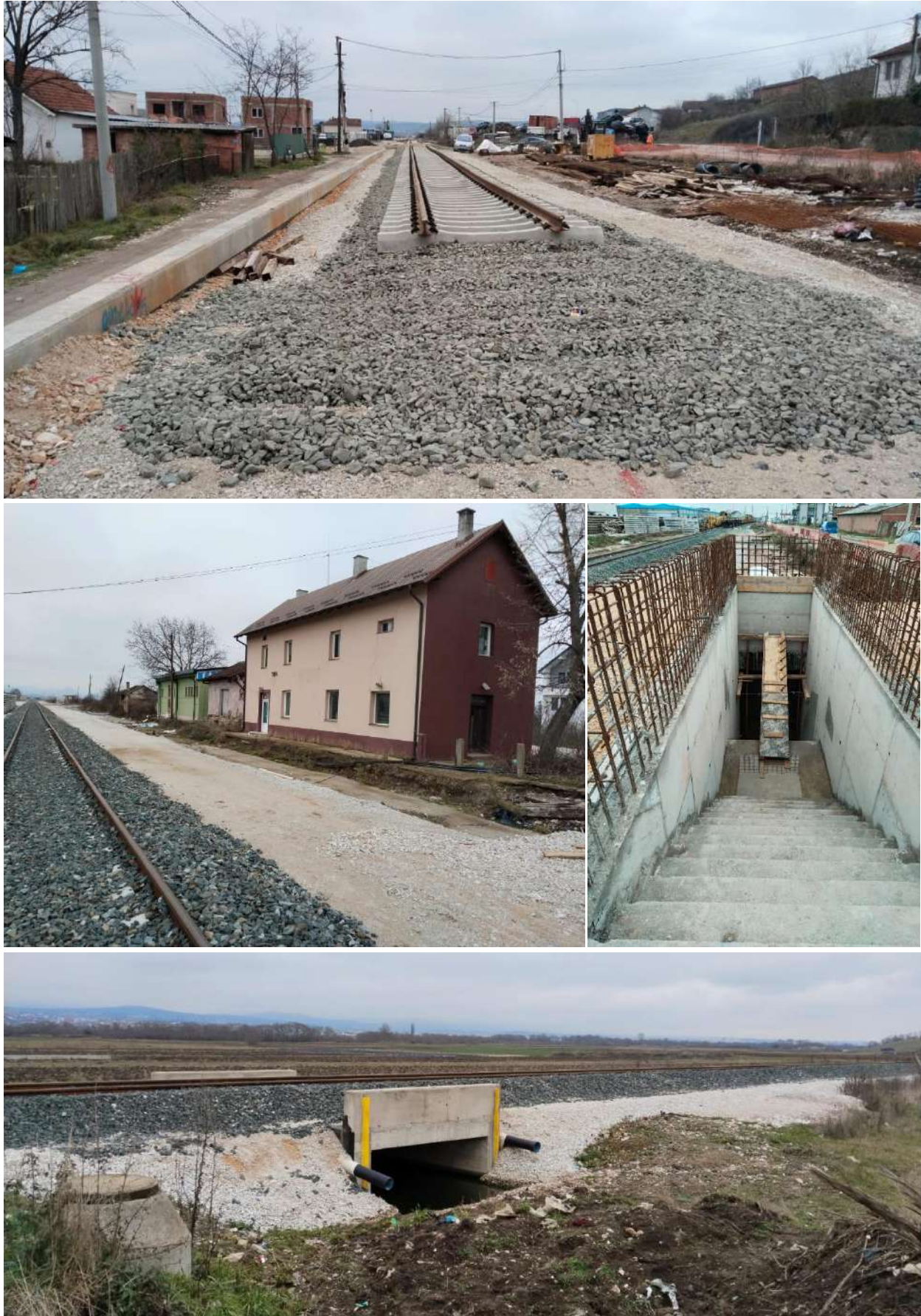
Station (platforms), track works, and culverts around Vushtri Station are progressing but not yet completed.
