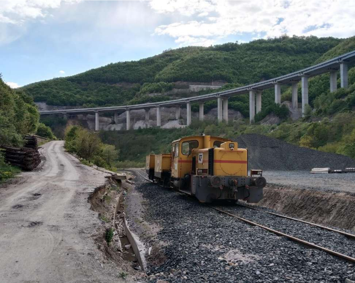
Views from the steel bridges and trackworks continued between Kacanik and Hani i Elezit stations along Phase 1 Works Contract.
